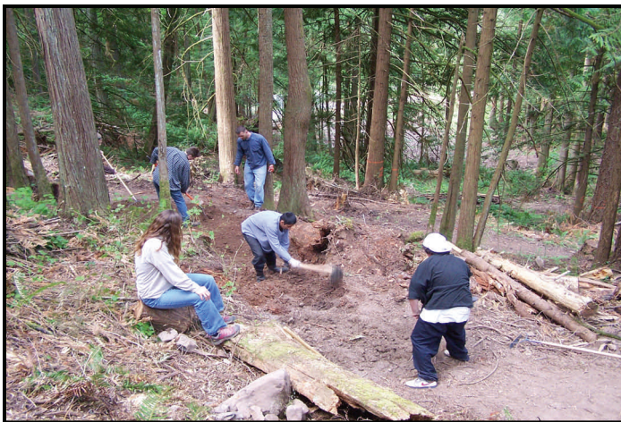
Parrot Creek Ranch trail crew realigned and surfaced a section of Hopkins Trail to make it an easier walk for more visitors to the forest.
