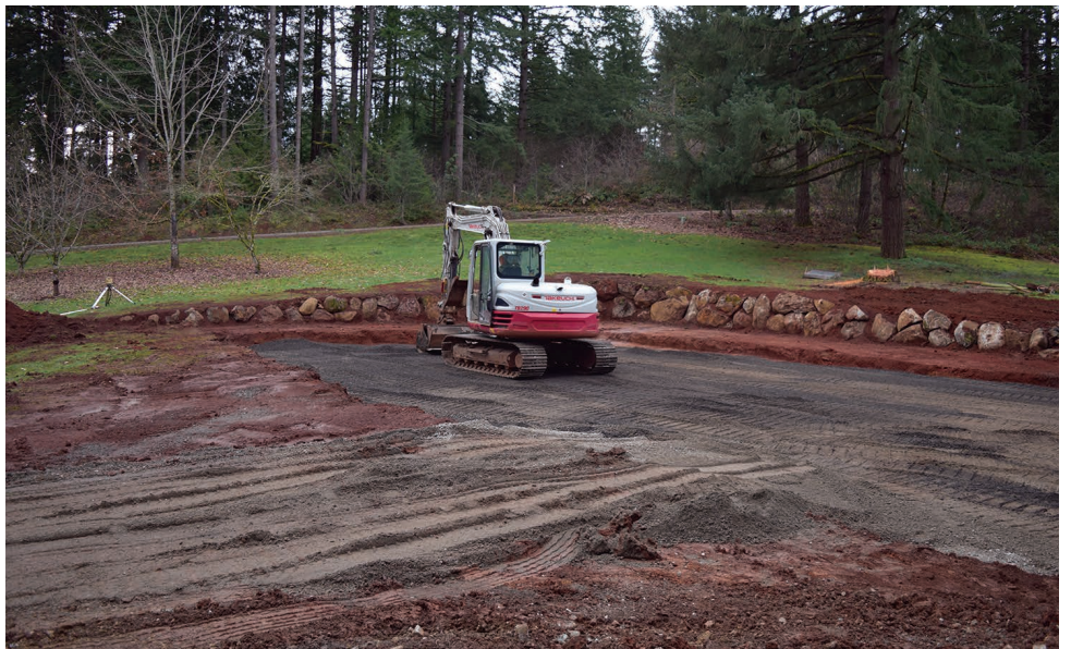
Great winter weather in late January provided the perfect time to dig out and level the site for the new Outreach Center.
