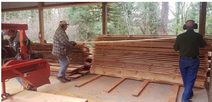
Volunteers milling cedar 1x12 lumber coming from Hopkins' trees for siding on the Outreach Center.
